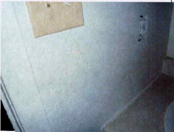
Wall Texture in Restroom
