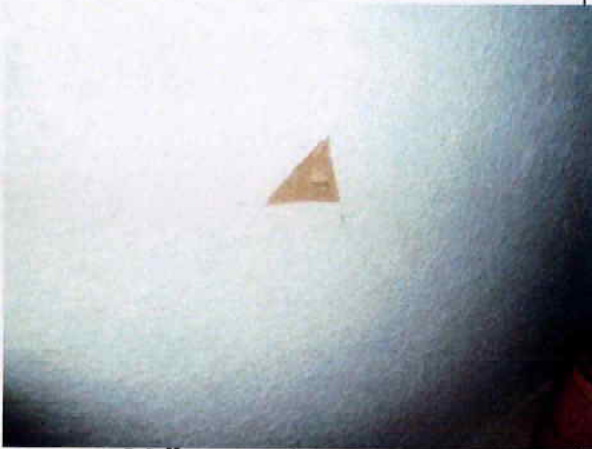
Wall Texture in Restroom
