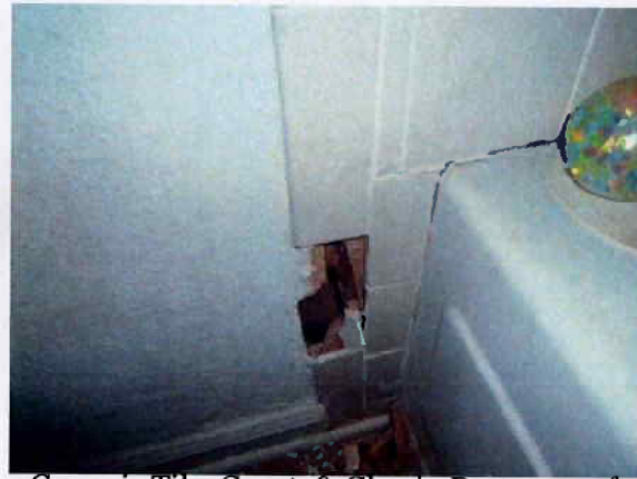
Ceramic Tile, Grout, & Glue in Restroom of
