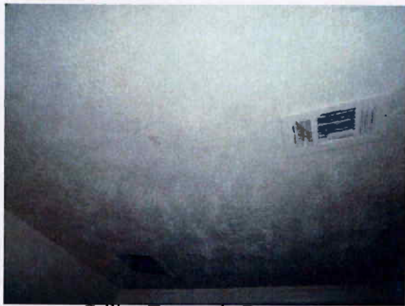
Ceiling Texture in Restroom
